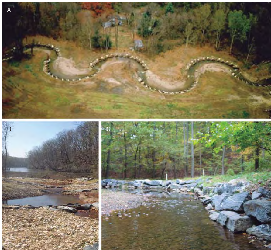
Figure 11.7: Channel reconfiguration is a broad phrase used to describe a host of restoration projects that involve a range of earth-moving activities. In extreme cases, this might involve completely reshaping the channel dimensions (e.g. width, depth, sinuosity, etc.) as in panel A) It may also involve creating a series of step pools B) that sequentially reduce the stream power and erosion in streams that have been incised due to deforestation, agriculture, or urbanization. Many channel reconfiguration projects include detailed design plans to protect stream banks from erosion C) and/or provide potential habitat for stream biota. (All sites located in Maryland, USA)
