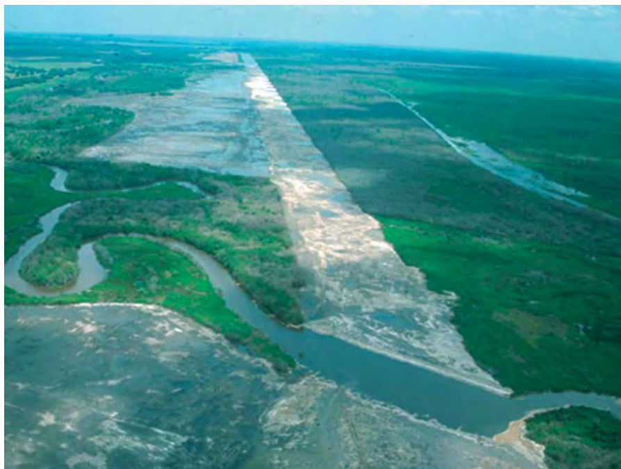
Figure 13.6: This photo, taken on February 9, 2001, shows the back-filled canal flanked by areas of degraded spoil. In the foreground, the remnant river channel has been reconnected across the back-filled canal to link up with an oxbow meander
